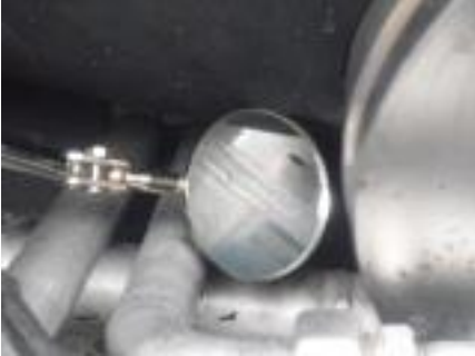
Photograph 4: Damaged weld seam
