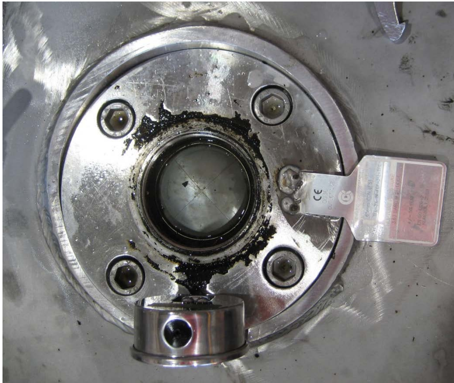
Picture 3: Separated identification plate of a bursting disk, welded onto the connecting flange of the safety valve
